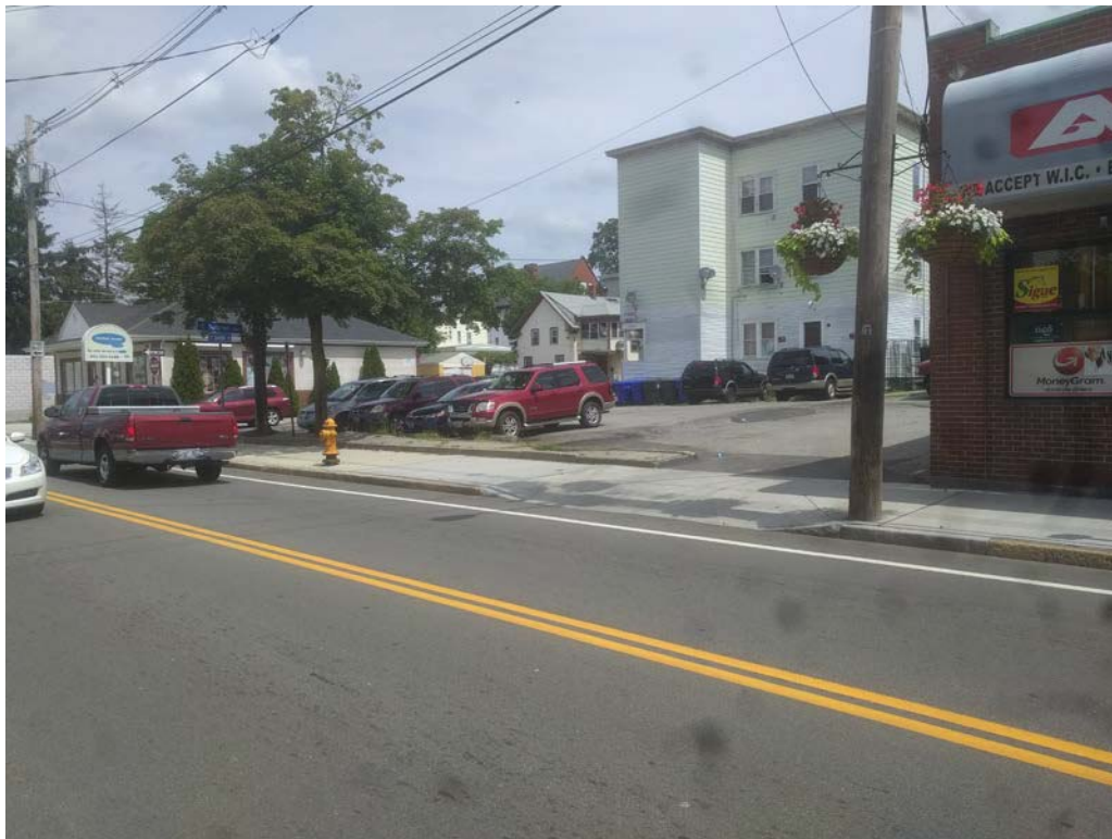
Lot 6-492 with depressed pavement at old building foundation
