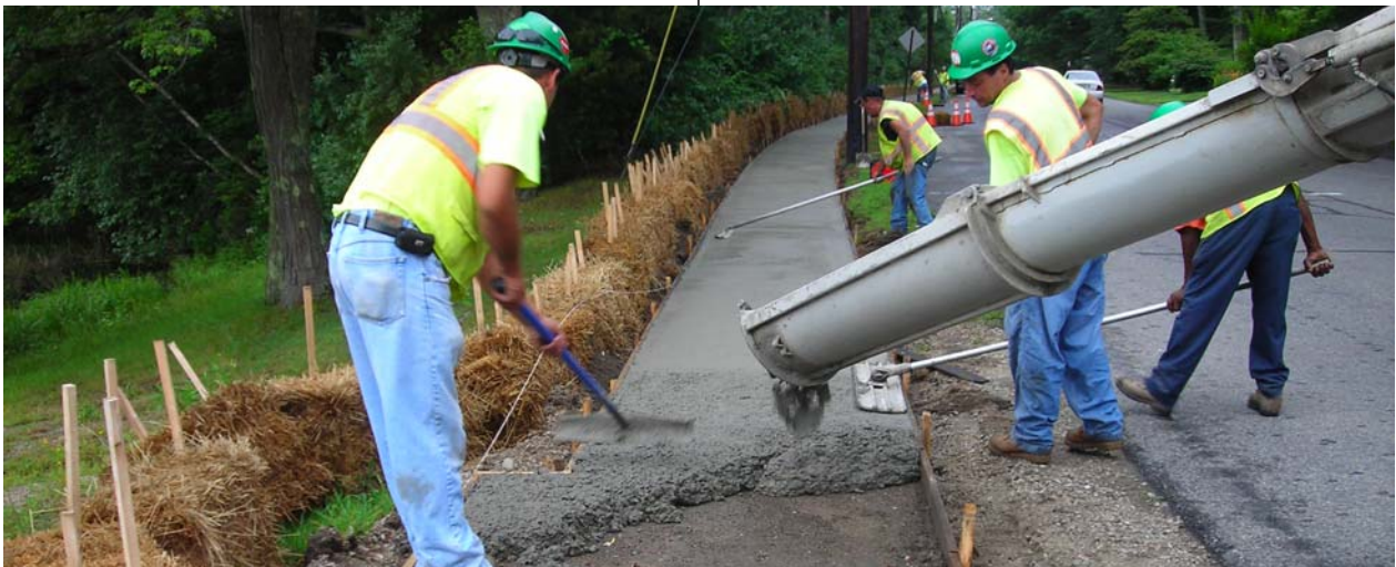
Sidewalk on Kent Street (2012) being built as part of a Safe Routes to School project for Hampden Meadows School
