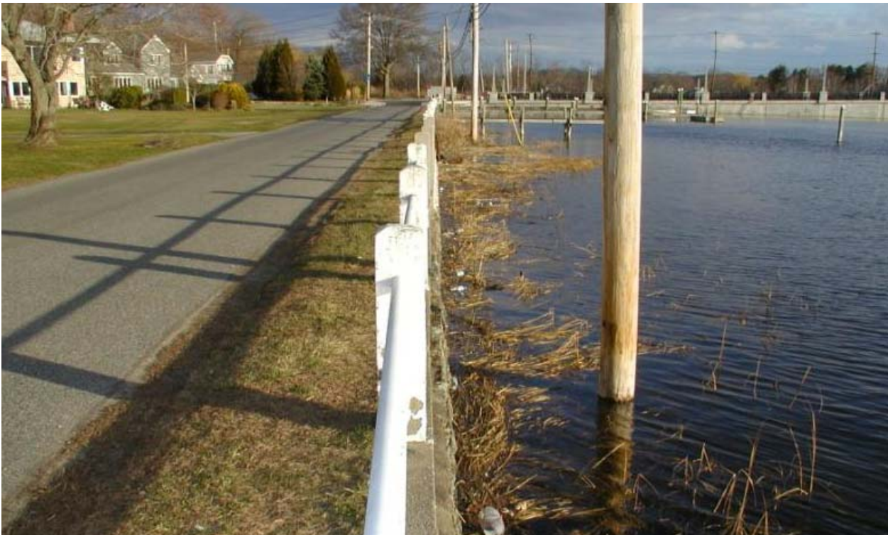
Figure 4. Adaptation Opportunity: Mathewson Road—Utilities
