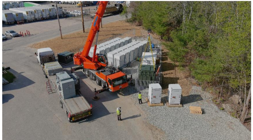
Pascoag Utility District Battery Storage (Agilitas Energy, 2022)
