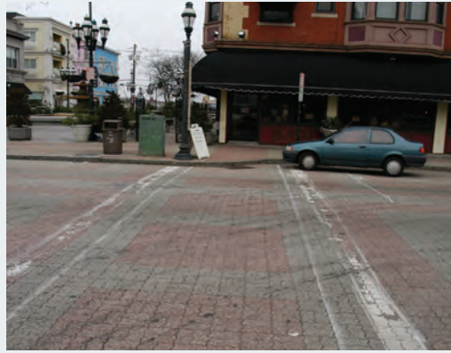
Pedestrian crosswalks were faded and inconspicuous
