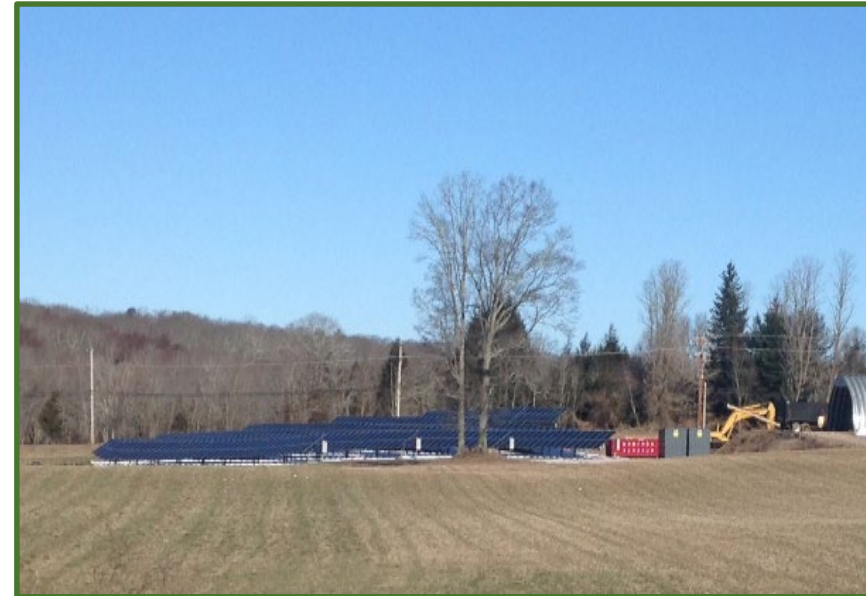
250 kW Solar Energy System, Reynolds Farm, Rt. 3, (between exit 1-2 along route 95) Hopkinton, RI
