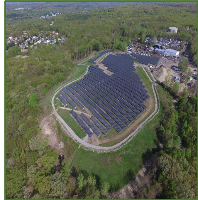
2.6 MW Solar Energy System, Closed Landfill. North Providence, RI
