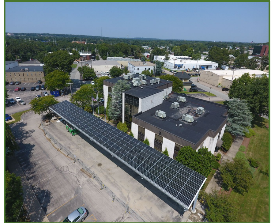
56 kW Parking Lot Canopy Solar Energy System - Public Utilities Commission Office, Jefferson Blvd, Warwick
