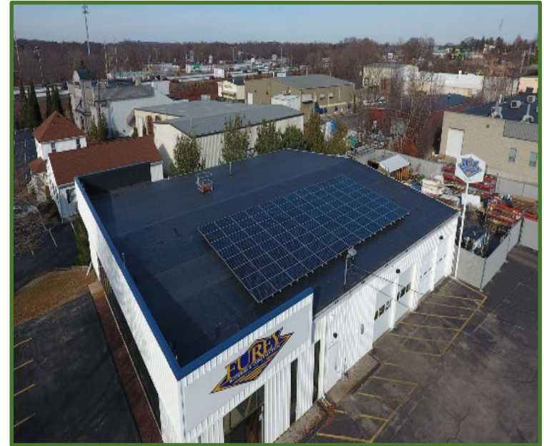
31.4 kW Rooftop Solar Energy System, Furey Roofing & Construction, Warwick, RI
