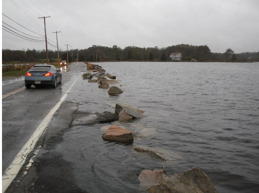
High tide flooding at Poppasquash Road
