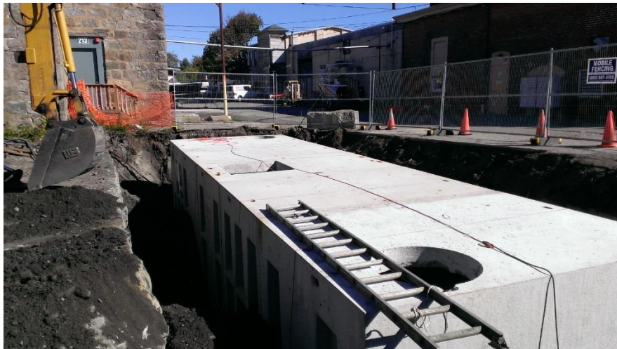
Stormwater BMP Sand Filter installed
