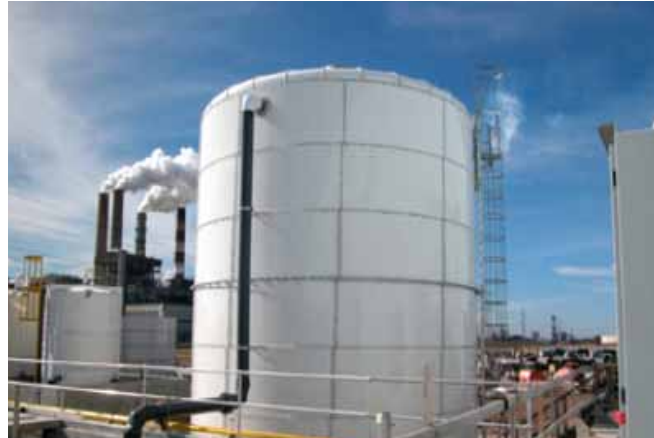
Tampa Bay Seawater Desalination Plant, Florida Source: http://www.water-technology.net/projects/tampa/
