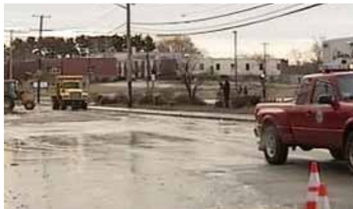
Water Main Break Pawtucket Avenue, East Providence, 2012 Source: Turn to 10, 01.06.12
